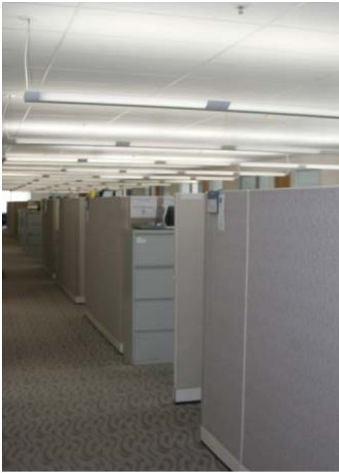
FIGURE 2: POST-RETROFIT Fluorescent pendants
