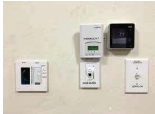
Figure 4. Manual control hardware in the IBCL.
