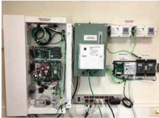
Figure 3. Automated control hardware in the IBCL.
